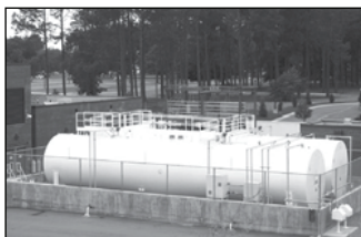
50,000 Gallon Dual Use Boiler / Generator
